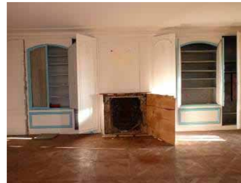
Figure 107 South West Bedroom, east elevation, showing hidden behind panelling and missing fire surround
