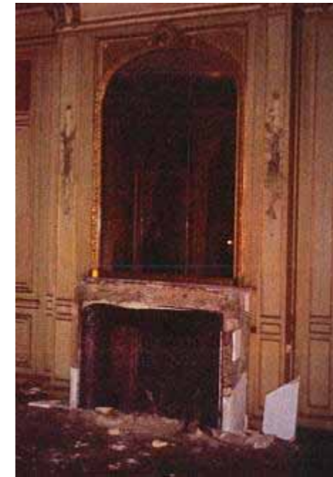
Figure 29 Drawing Room, fireplace surround missing but remnants of original mantel and mirror remain
