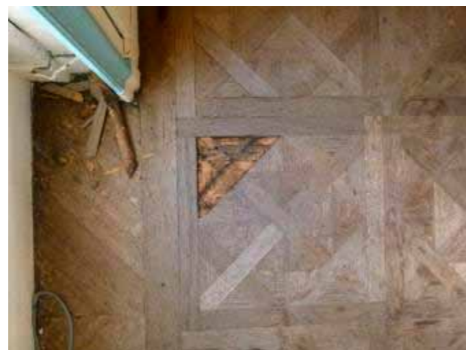
Figure 105 South West Bedroom, showing damage to parquet flooring
