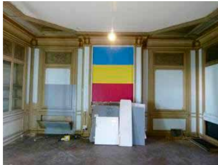
Figure 14 Drawing Room, east elevation, showing over painting and open panel
