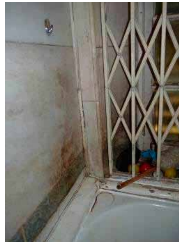
Figure 95 Bathroom, dirt and deep staining to marble in south west corner above bath near window
