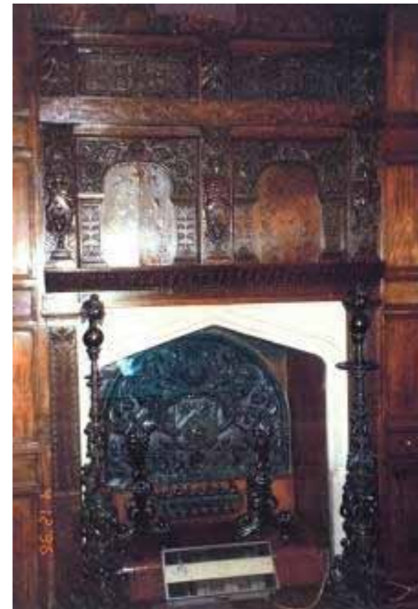
Figure 40 Dining Room, detail of fireplace in original condition with carved timber surround and wall panelling
