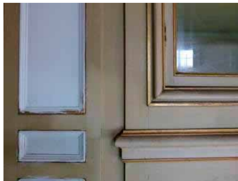
Figure 28 Drawing Room, area of wall and gilding cleaned, gilded beading appears brighter
