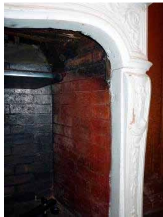
Figure 87 North West Bedroom, detail of fire surround showing over-paint
