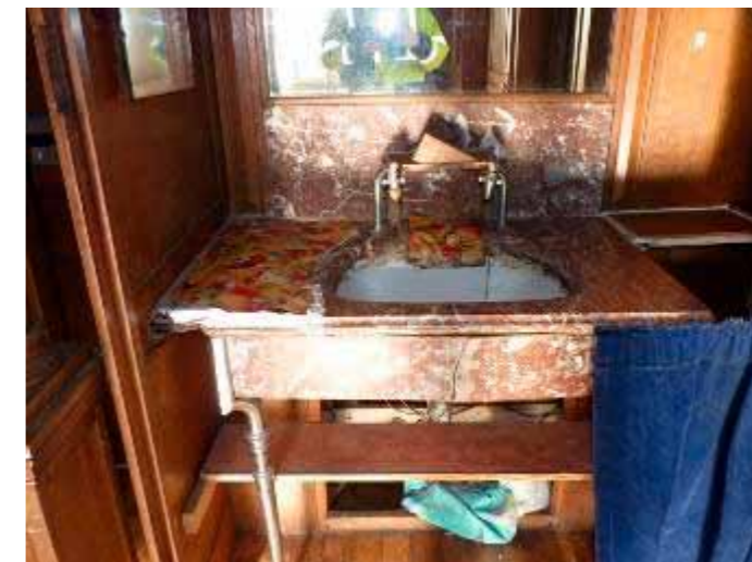
Figure 81 Normandy Bedroom, detail of damage to marble wash area
